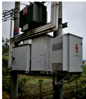
Southern Power Grid Cooling
