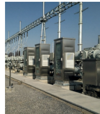
State Grid Cabinet Cooling
