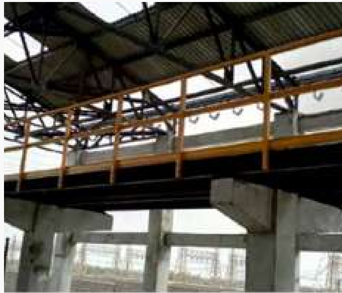
Fiberglass Handrail & Stairway
