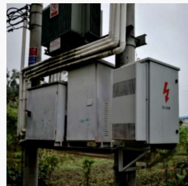
Southern Power Grid Cooling
