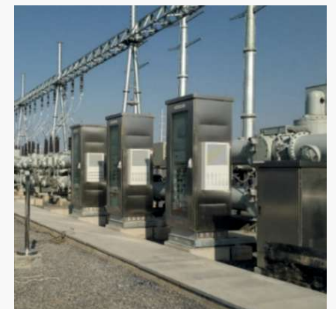
State Grid Cabinet Cooling
