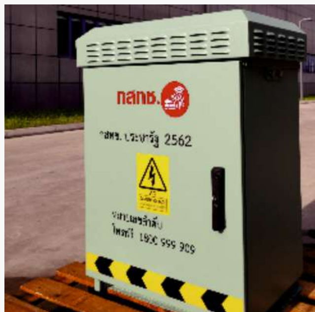
Thailand Cabinet Project
