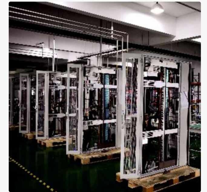
In-row Aircon For Germany Customer
