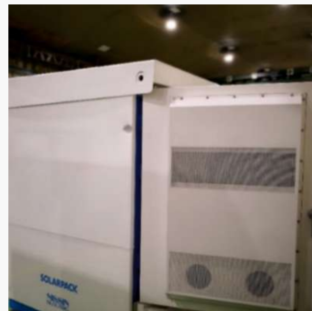
Nissin Energy Inverter Cabinet Cooling
