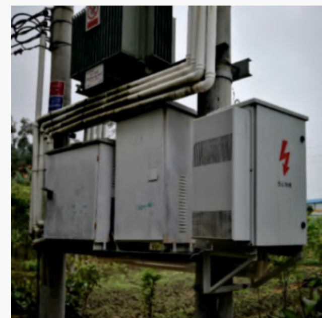
Southern Power Grid Cooling
