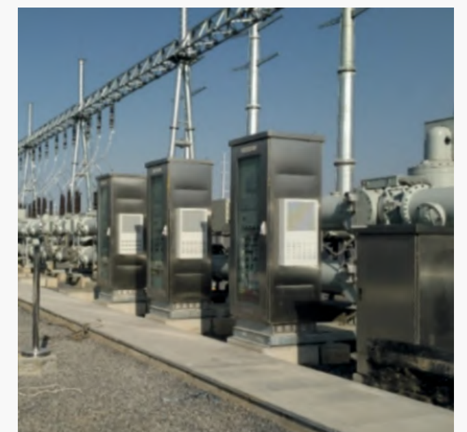
State Grid Cabinet Cooling
