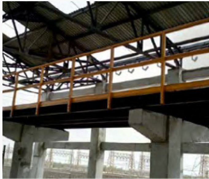
Fiberglass Handrail & Stairway
