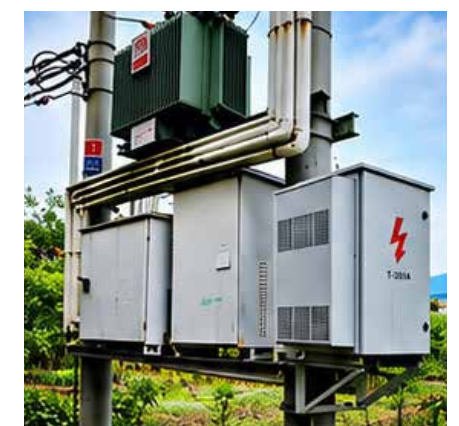
Southern Power Grid Cooling
